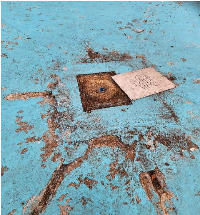
Photo 1 – Screed and Paint breakdown around drain
