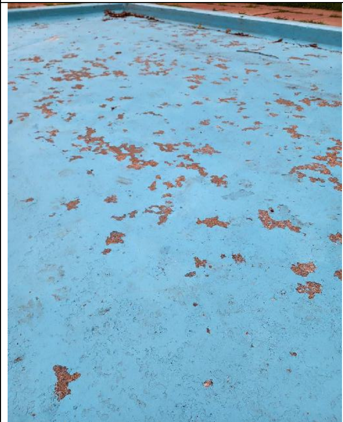
Photo 5: Delaminated paint throughout the pool tank
