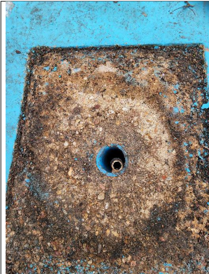
Photo 9: Central drain without cover over
