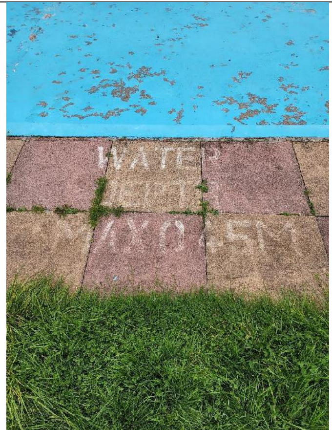
Photo 14: Painted markings to paving slabs - Faded
