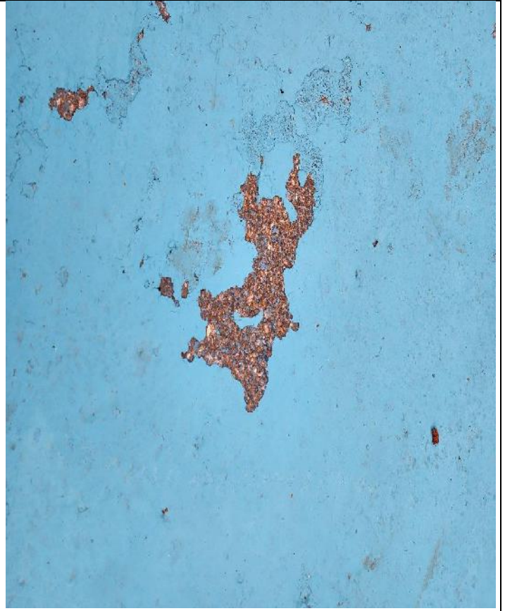
Photo 8: Example of paint delamination with screed below
