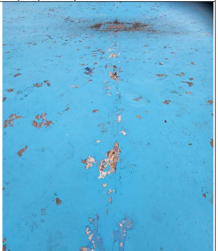
Photo 6: Pitting and delaminated paint example
